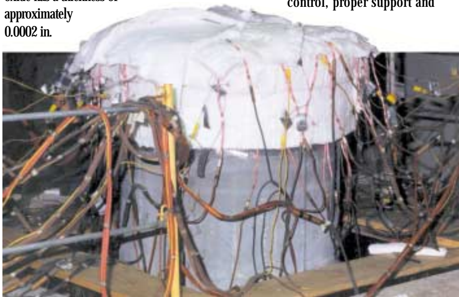
In-shop heat treatment of Zr702 tube welds and tubesheet for a heat exchanger. Photo courtesy of Phoenix, a division of Kodiak Industries Inc.
