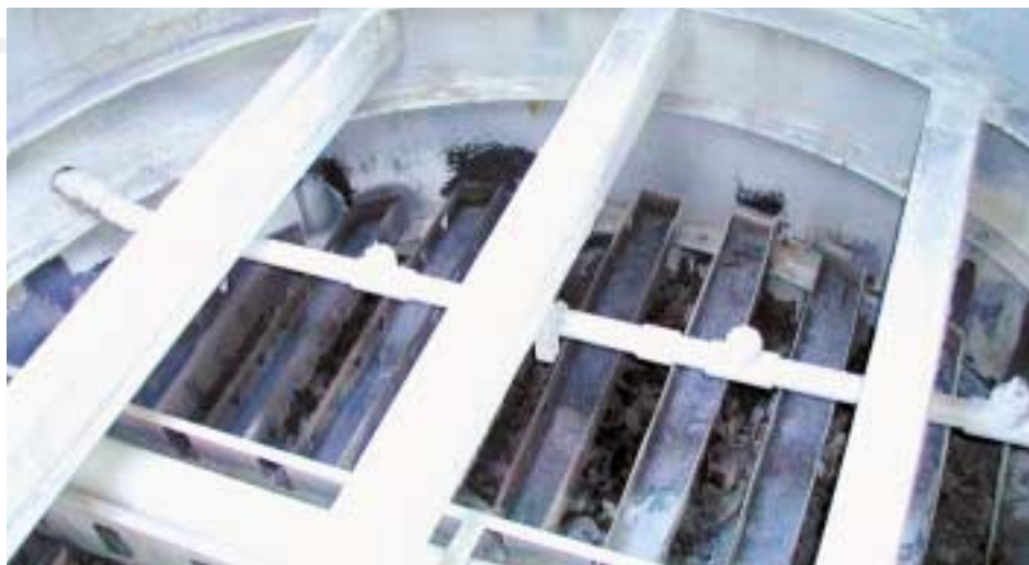
Figure 2. Zirconium in caustic scrubber—no corrosion after 15 years of service.
