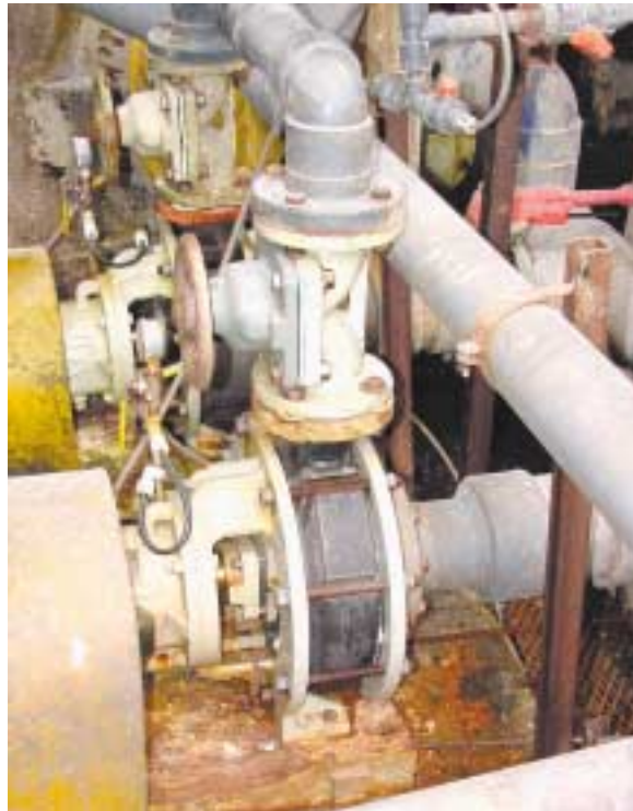
Figure 1. Zirconium Recirculation Pumps on Water Scrubber
