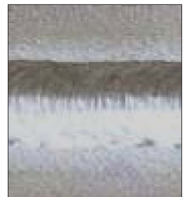
Figure 1. Bright band along weld toe is caused by welding heat
